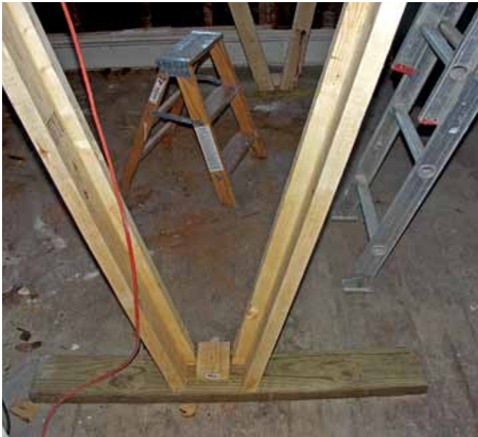
During the work, V-shaped supports propped up lateral temporary shoring; the system was moved daily to access new work areas.
