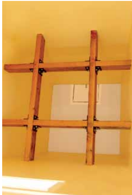
Atop the finished tower's interior, 4x8 collars placed horizontally (and plated and through-bolted) add extra support.
