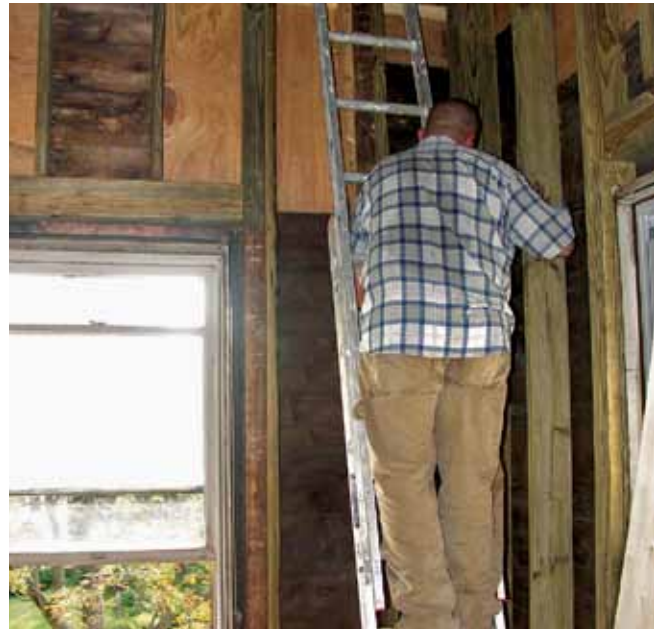
Installing new framing and sistering beams were critical to shoring up the tower.
